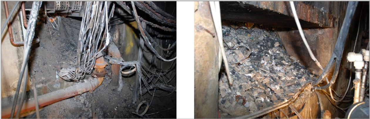
Figure 19 – Cables exiting vertical ducts into level 2 Plenum
